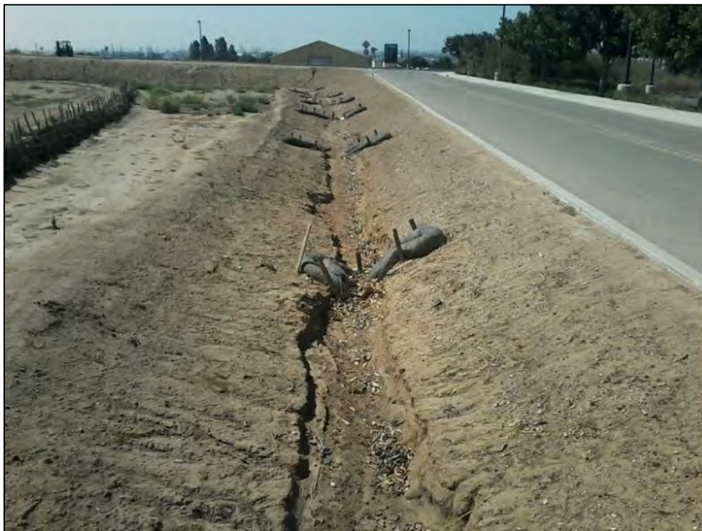
PHOTO 18. DRAINAGE LOCATED ALONG BIRCHKNOLL ROAD, FACING SOUTH.
