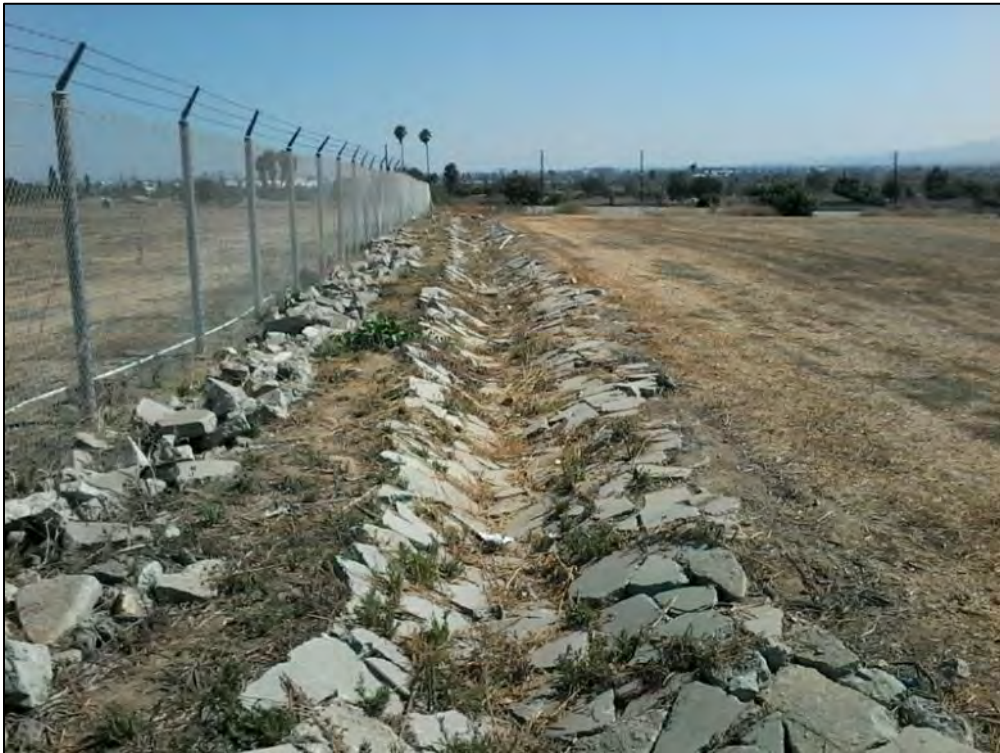
PHOTO 22. CONCRETE LINED DRAINAGE LOCATED ON WEST SIDE OF MAINTENANCE FACILITY, FACING SOUTH.
