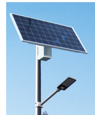
Exhibit 6-9: Example of LED and PV Powered Site Lighting
