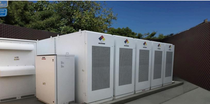
Exhibit 6-5: Example of battery storage
